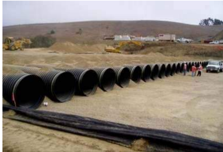
2 Million Gallon Storage & Re-use System (Cambria School, CA)
