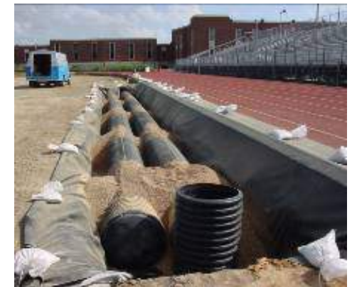
5,000 Gallon Regulator Tank (SMU, TX)
