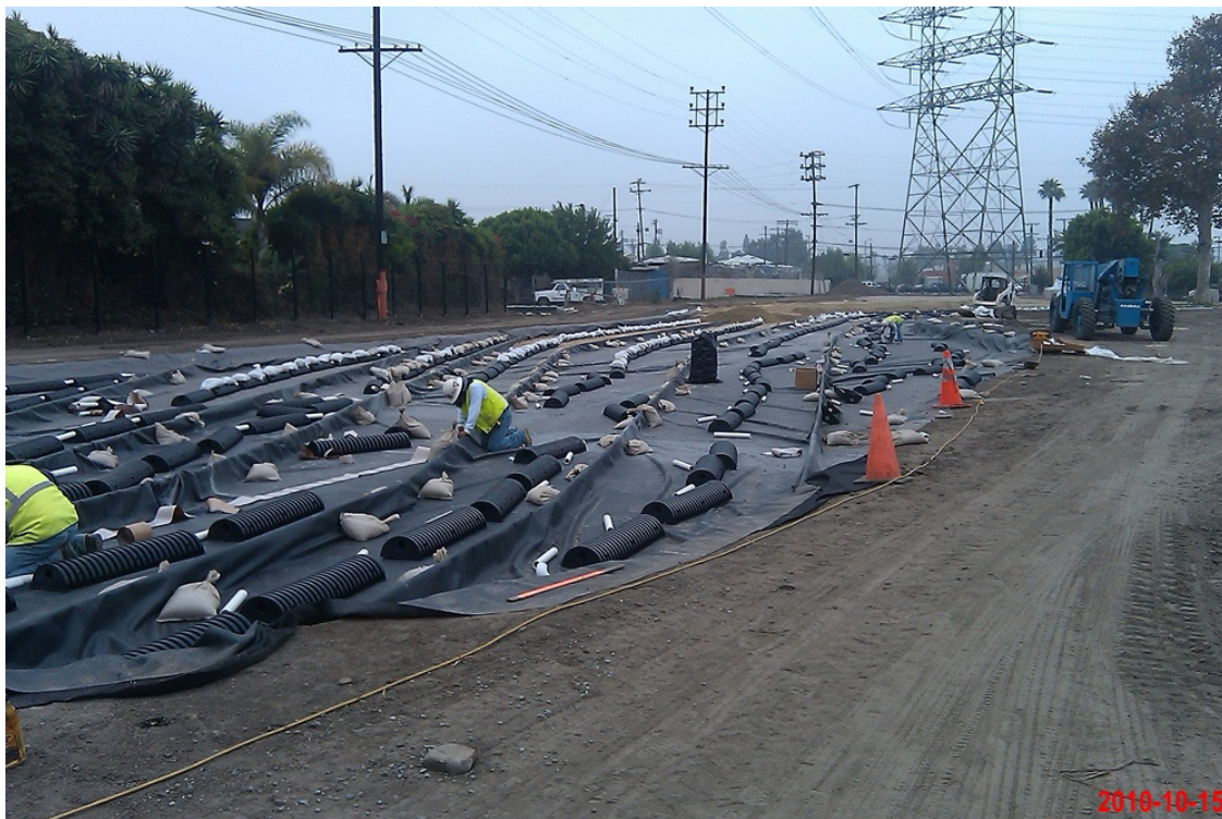
Photo was taken on October 2010. Picture of the installation of the infiltration system.
