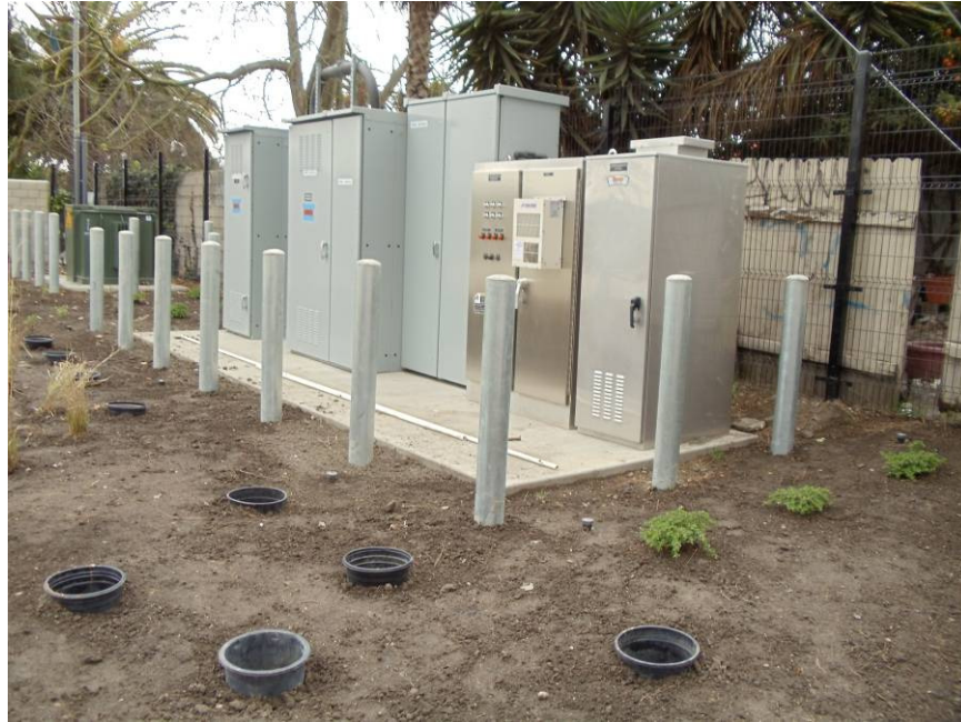
Photo was taken on February 2011. The lift station control panels at the site.
