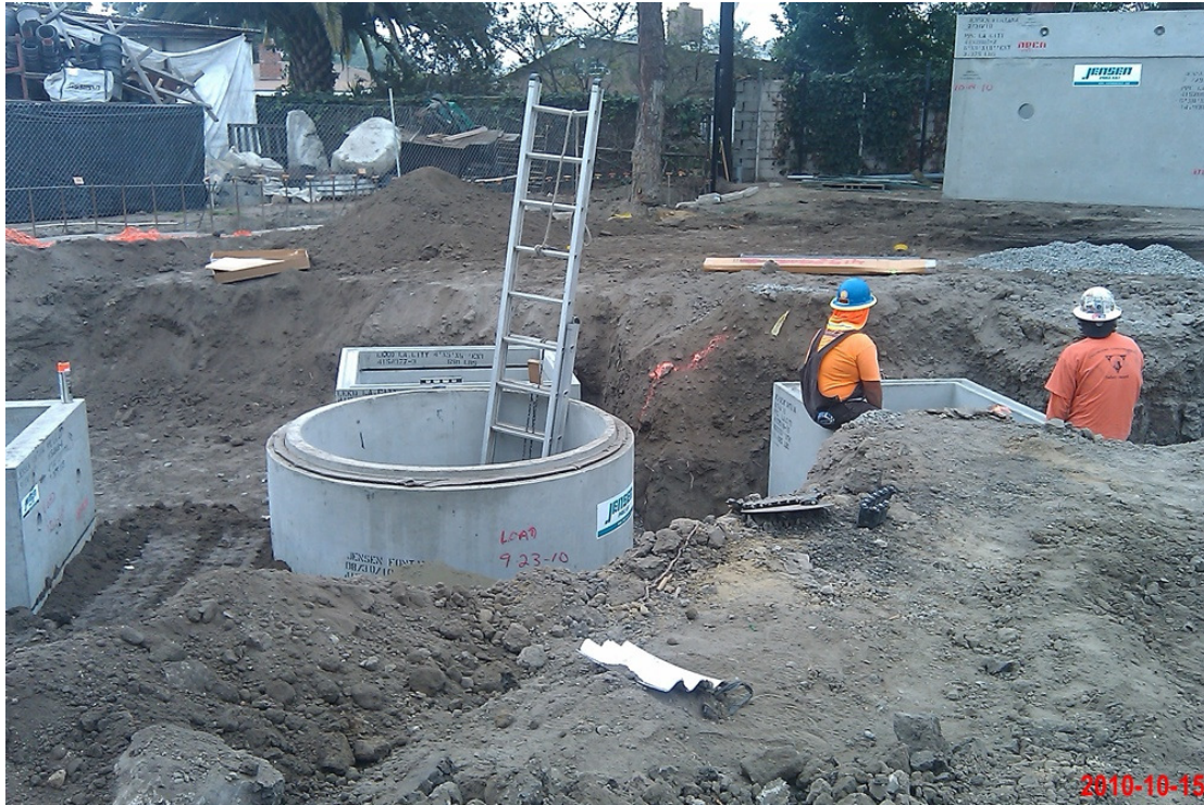
Photo was taken on October 2010. Picture of the pumping station and treatment train installation.
