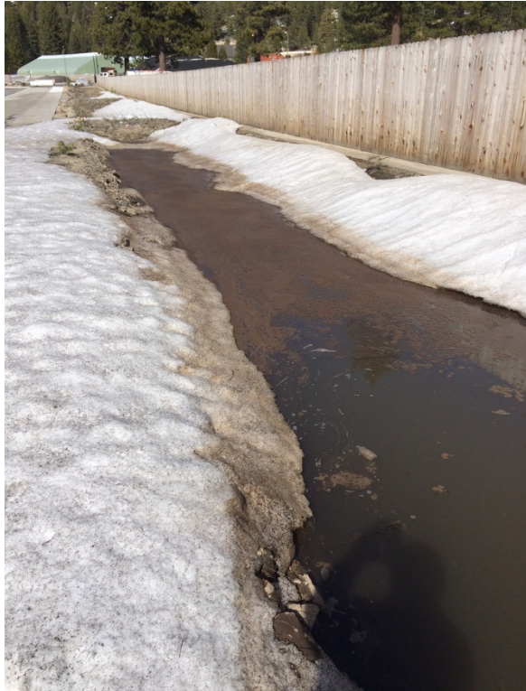
Fig 9. Adjacent Infiltration basin BMP
