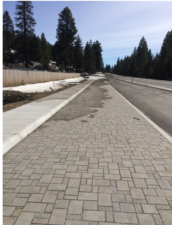
Fig 10. Basin overflows onto EPIC profile
