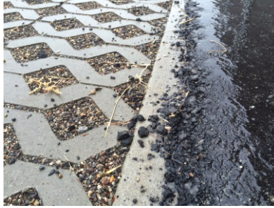
Asphalt deposits retained at surface
